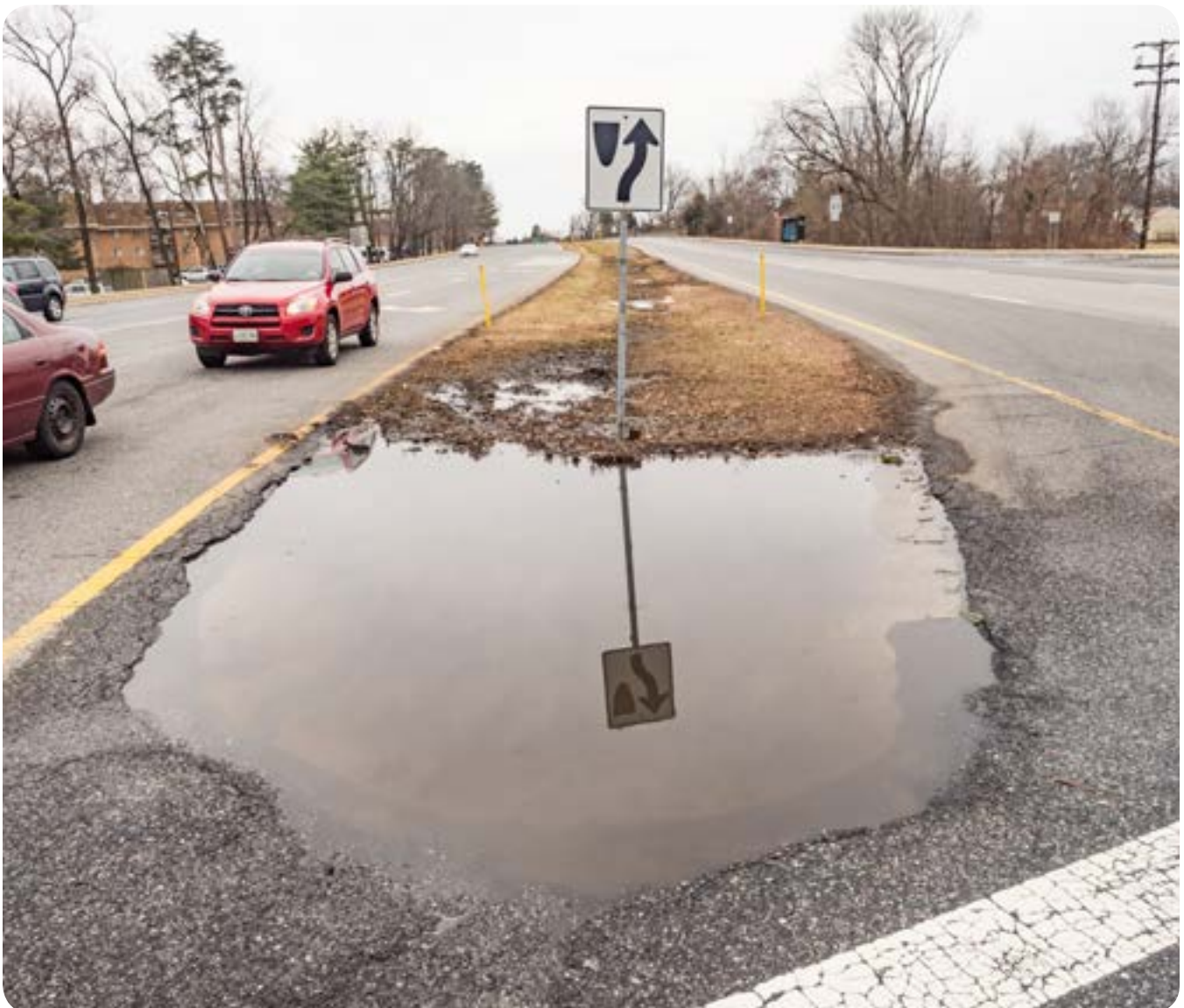
The median at Georgia Avenue and Bel Pre Road is typical of a medians in the Aspen Hill area: they are not protected and may present barriers to people with mobility devices, strollers, and low or no vision. Refuge islands provide a safe space for people to rest or wait while crossing the roadway and may also be used for stormwater management.
